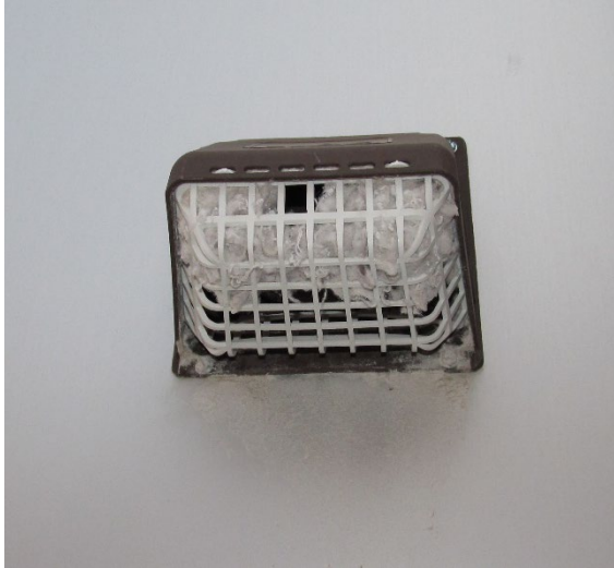
Figure 4. Note the potentially dangerous lint build up on this screened dryer vent.
